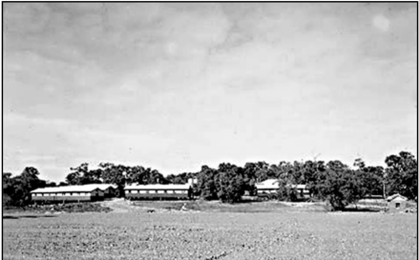
Leeuwin's parade ground and sports fields under construction. In the background are the original accomodations blocks or 'dongas' (RAN)
