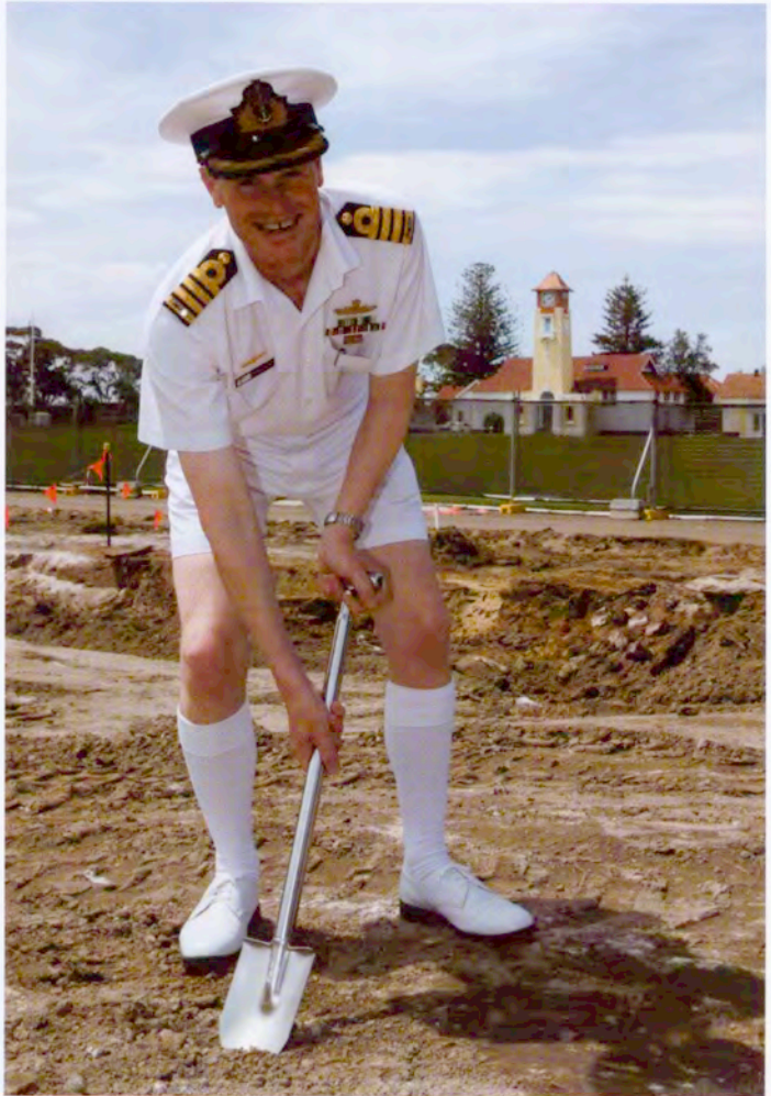
Captain Vandyke turns the first sod ceremoniously for the new Geelong House
